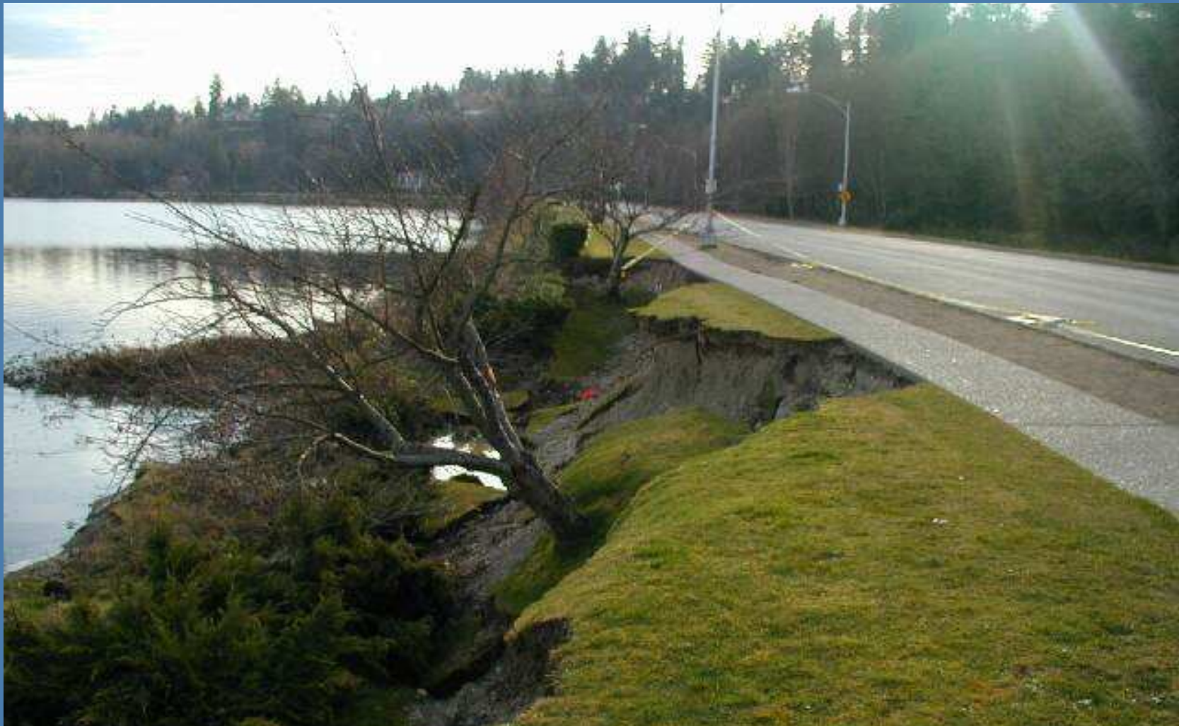
Capital Lake, Olympia, Washington (Nisqually event, 2001) Lateral spreading from magnitude 6.8 earthquake
