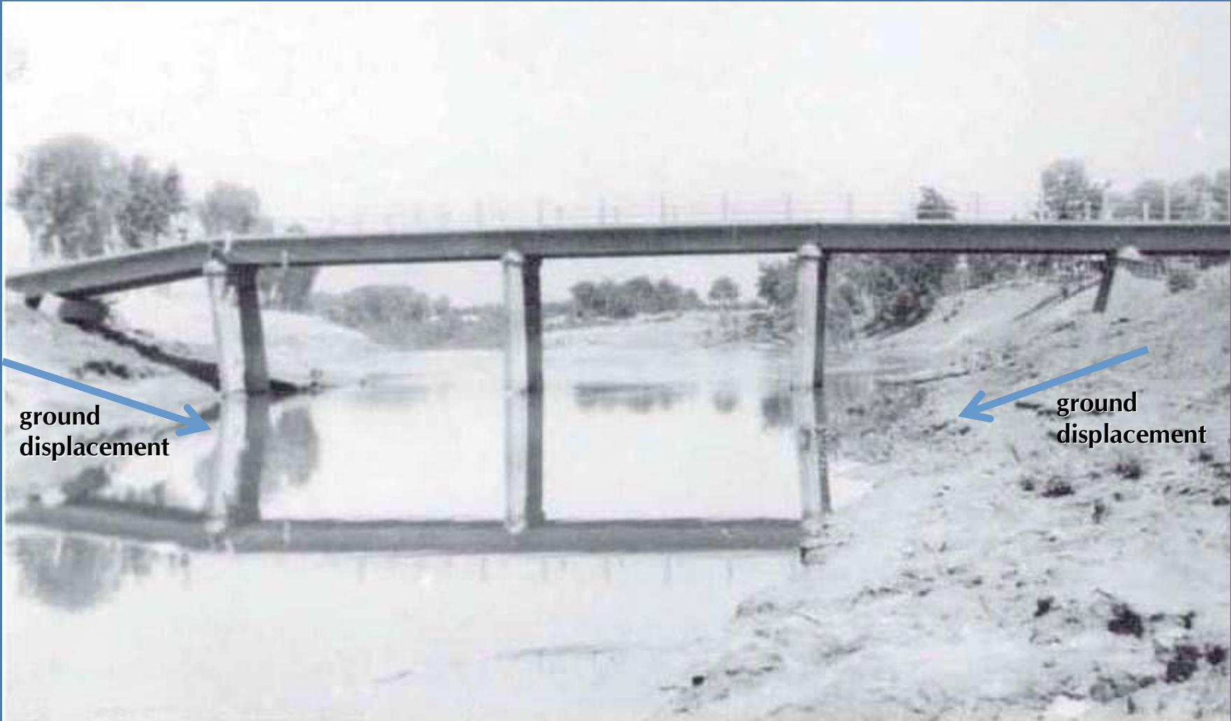
1976 Tangshan Earthquake - Yuehe Bridge near Tangshan, China (M7.8 earthquake)
